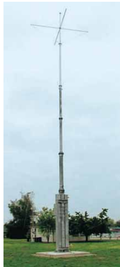
Abb. 4: Beacon-Sendemast in Iffezheim (293,5 MHz).
